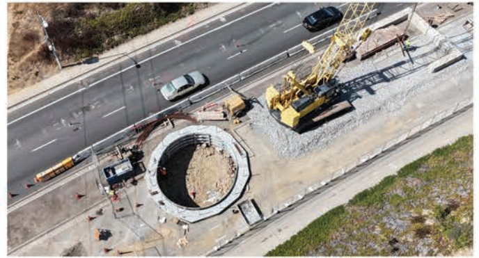
Ongoing excavation of third tunneling shaft on Genesee Avenue north of Rose Canyon
